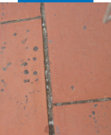
An example of old terracotta floor requiring treatment before applying Aquaflex Roof
